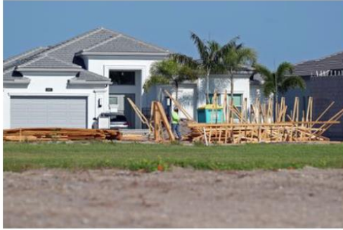
A construction worker walks through lumber at Valencia Sound in Boynton Beach on May 24, 2021. The development is being overseen by GL Homes. (Amy Beth Bennett / South Florida Sun Sentinel)
